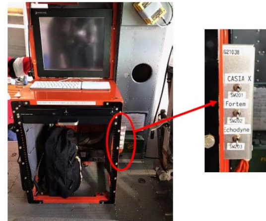
Figure 3. Engineering Workstation power switches
